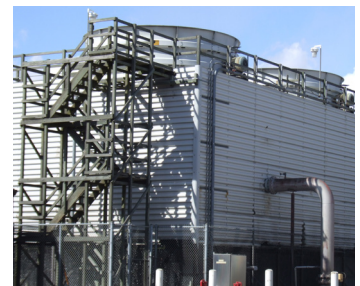
The cooling tower turns steam back into water.
