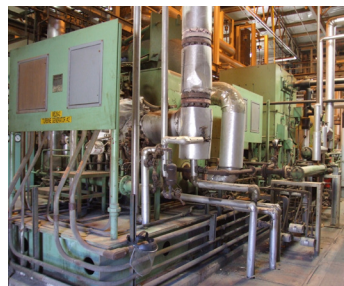
Steam drives a turbine generator to create electricity.
