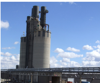
Sawdust is ground and stored in three main silos.
